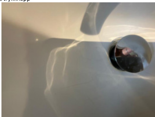
Riss i servant
