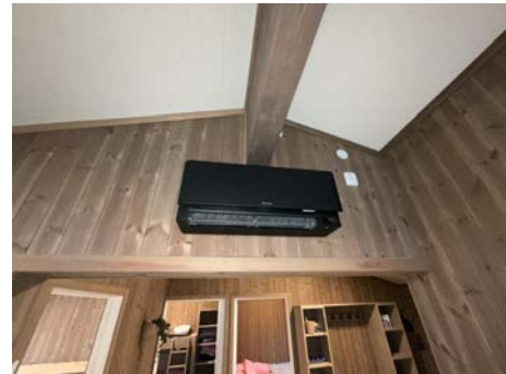
Varmepumpe, innvendig aggregat.
