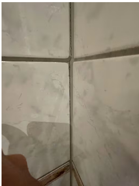
Sprekker i fuger.
