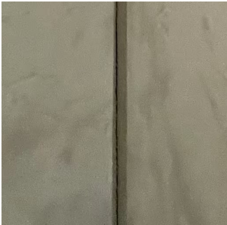
Sprekker i fuger.
