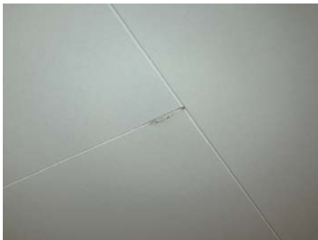
Fuktsvelling i himlingsplate
