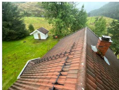
Stigetripp ok men mangler snøfanger.
