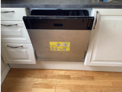
Oppvaskmaskin mangler front
