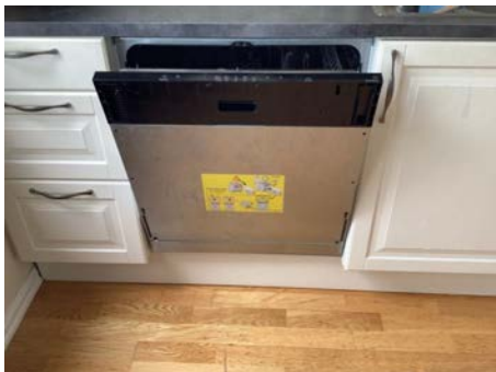
Oppvaskmaskin mangler front
